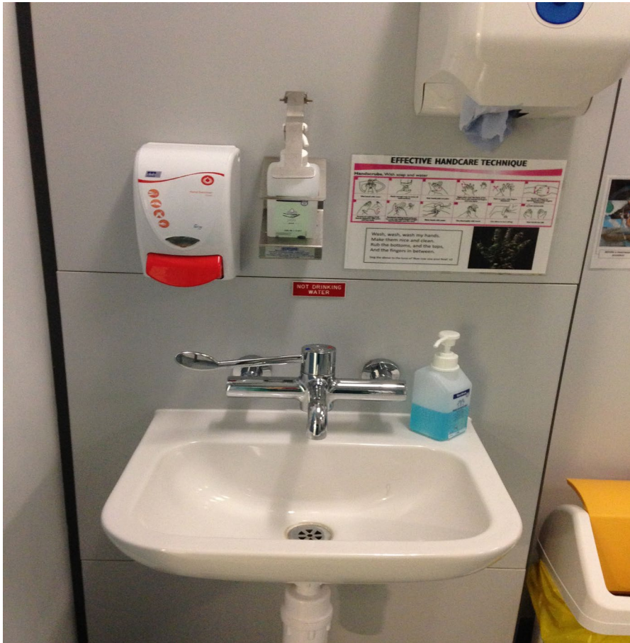
▲ Figure 2. An example of a hand-washing station
